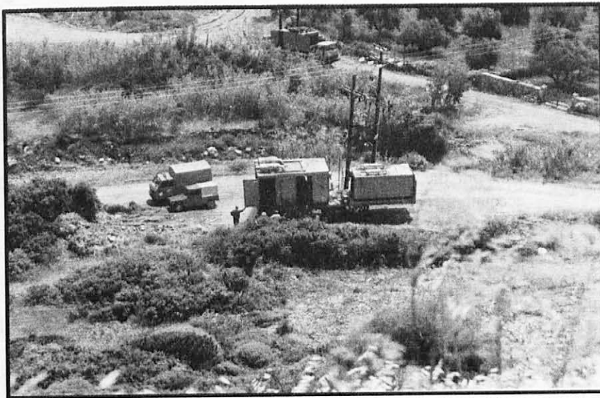
THE GENERATOR AT AGIA PATRICIA
